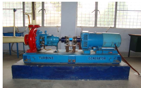
Fig. 3: Tested centrifugal pump coupled with generator
