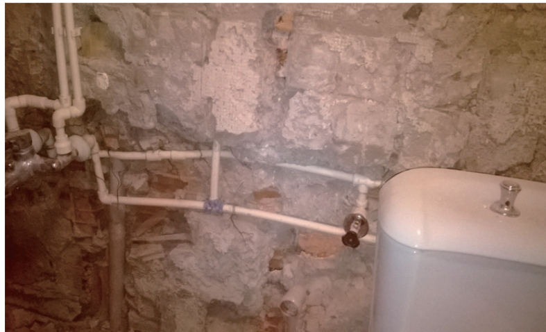
Figure 5 Views From the Repair Works in the Bathroom of a House Bought Second Hand at a Fairly Cheap Price (Photo: Courtesy of Geography Teacher F. GÜNDAR, A Relative of the Author)
