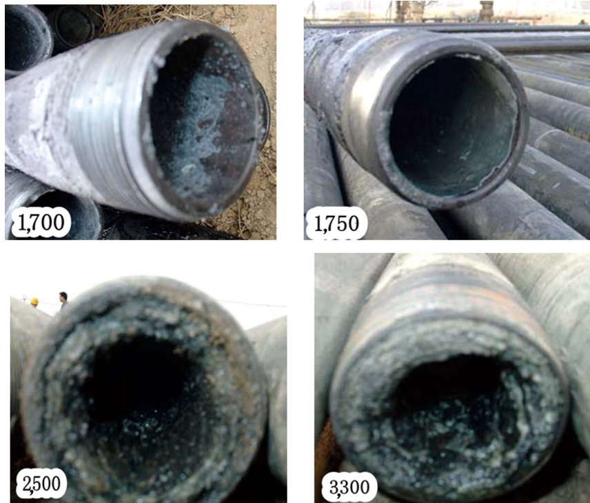
Figure 1 The Scaling in Water Injection Pipe at Different Well Depth
